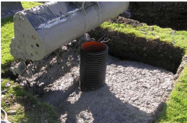
Installation with sockets
