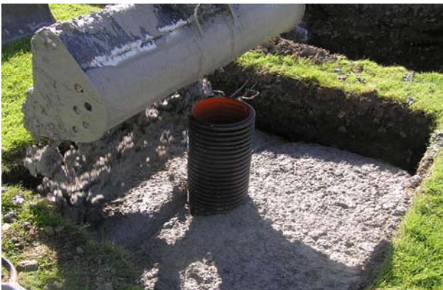
Installation with sockets
